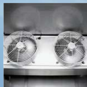
Blower pressure monitoring
